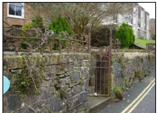
Maintenance problems, High St (top), lost ironwork, Combe St (above)
